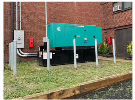
A new generator at the Department of Public Works Yard complex
